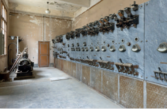
7. A modern heritage: the electrical transformer (1931-1932) and its preserved interiors © Patrice Giraud, Inventaire général, Région Pays de la Loire.
